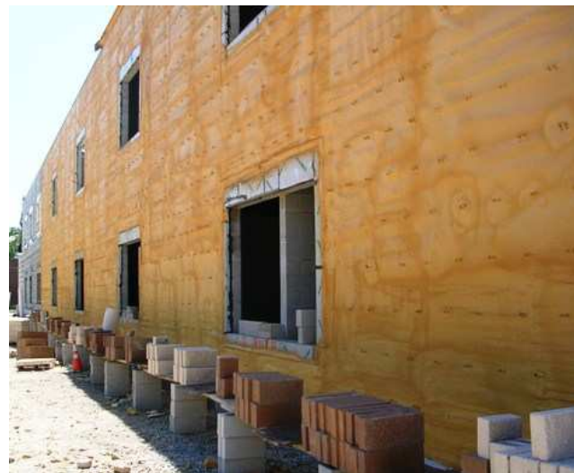
Maple Heights High School. Work Performed by Giambrone Masonry and members of Local 5 Ohio Administrative District Council. Product: NCFI Insul
